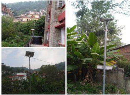
Girls Hostel Solar Lights
